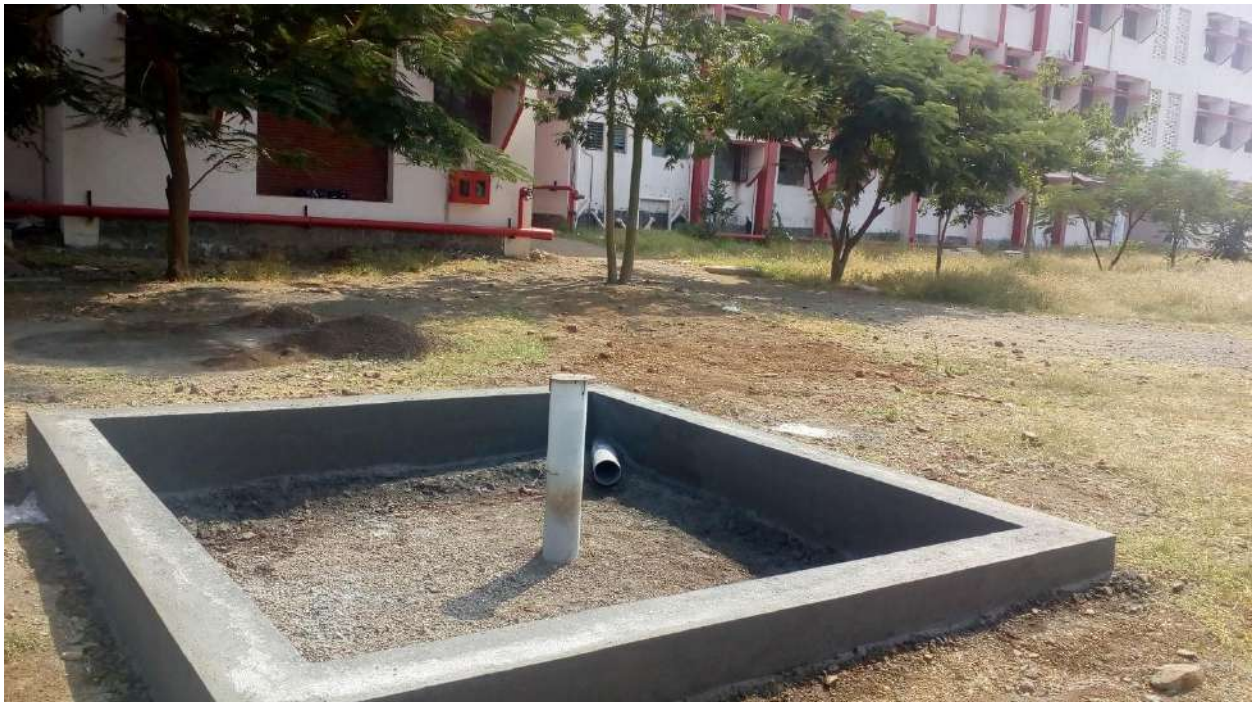
Fig: Rain Water Harvesting system
