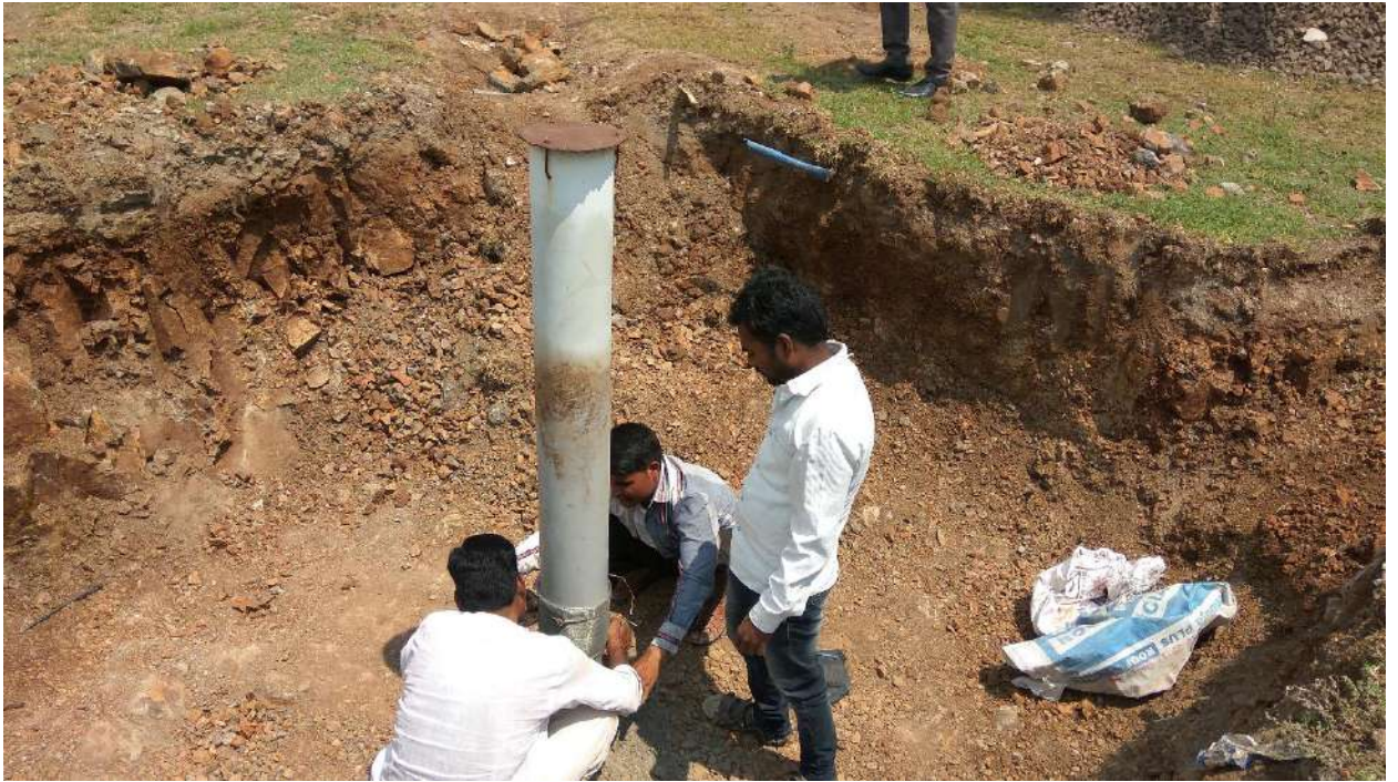
Fig.3: Meshing to recharge holes of bore well pipe
