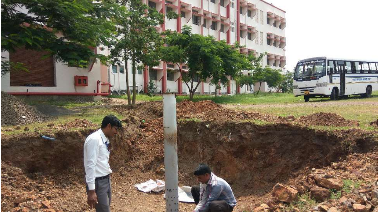
Fig. 2: Recharge holes to bore well Pipe
