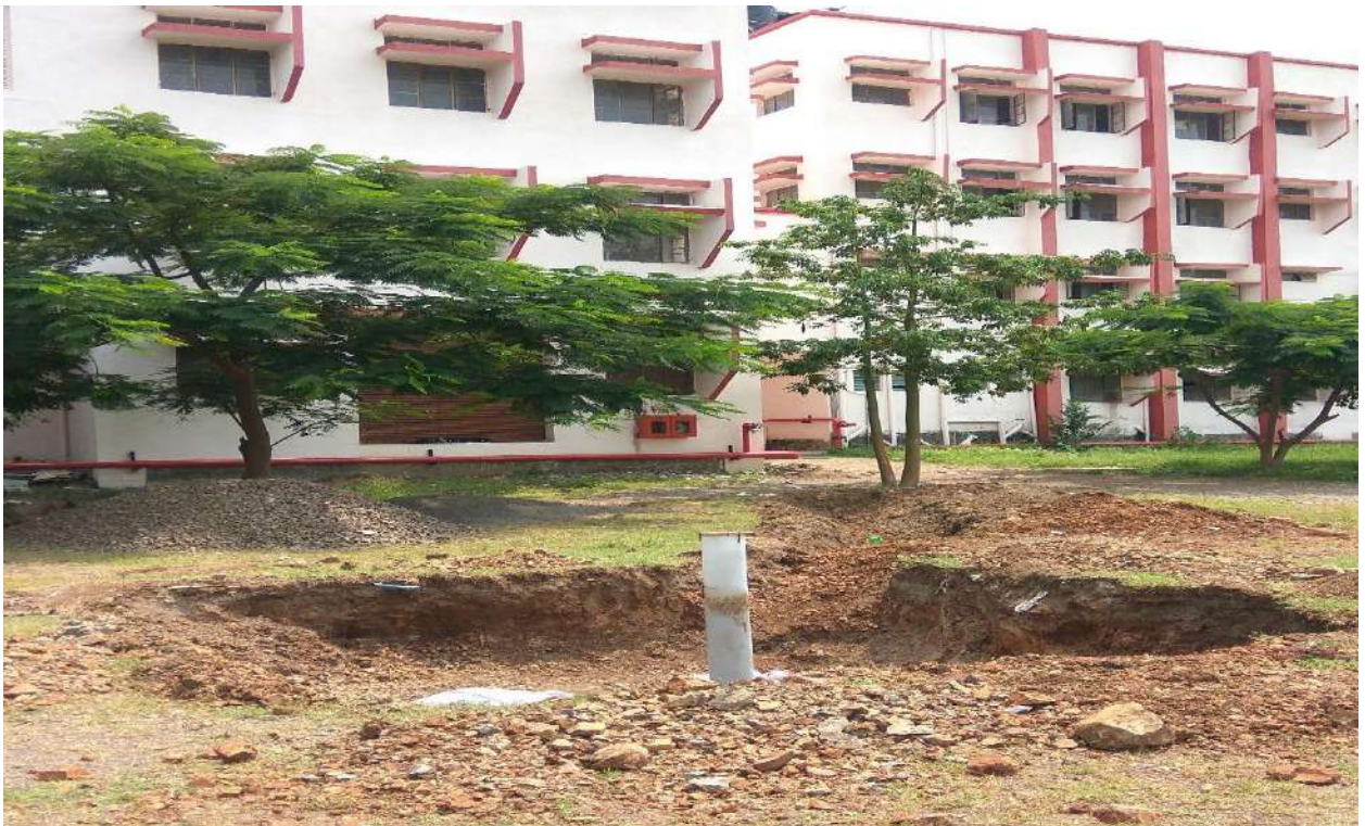
Fig. 1: Rain Water Harvesting Filtration Unit Ditch
